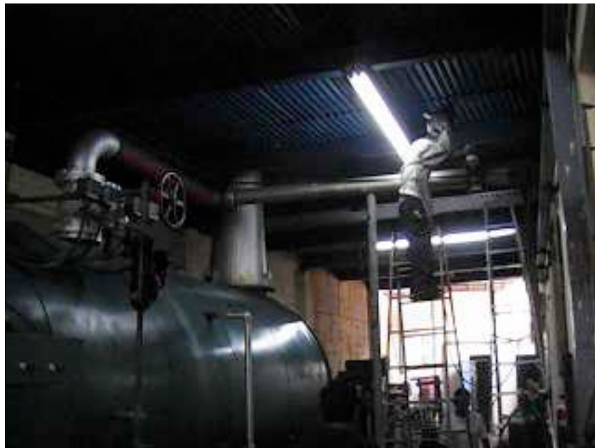
400 hp Cleaver Brooks Boiler in El Salvador
