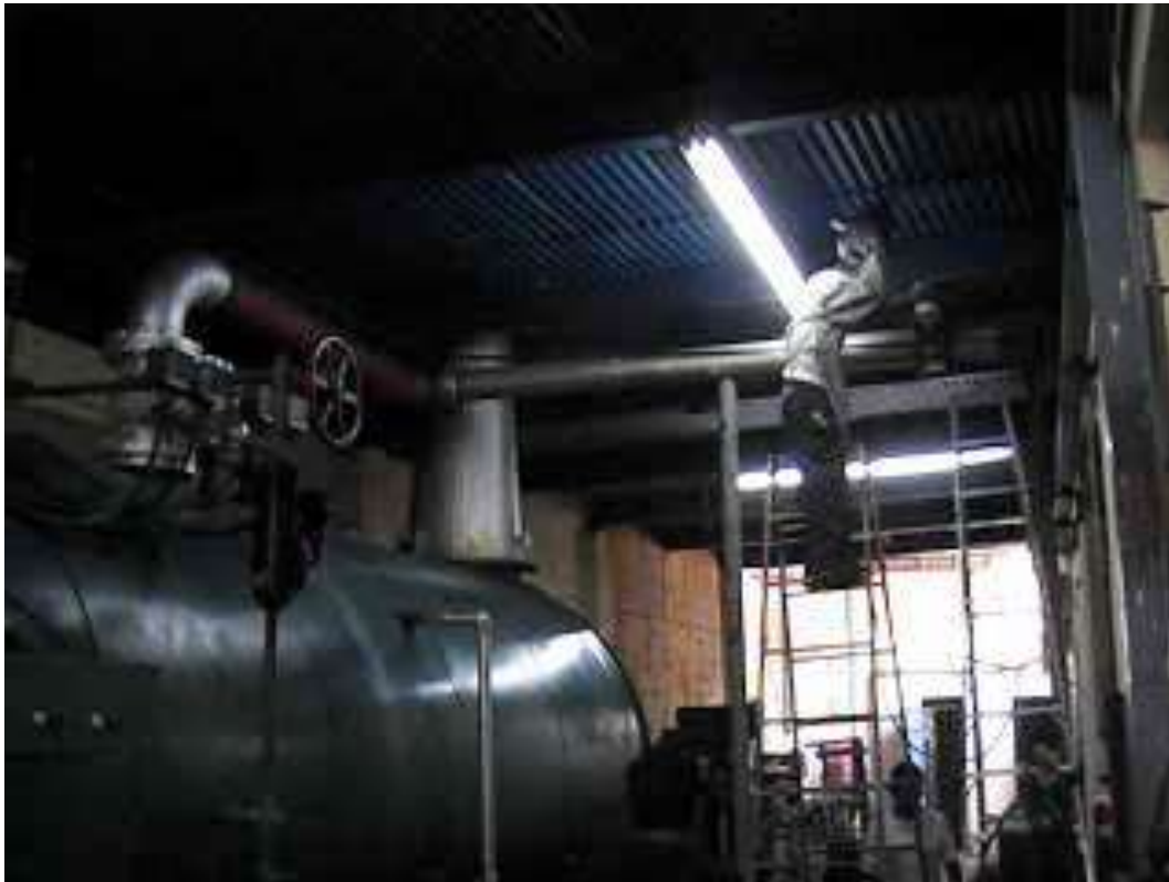
400HP Cleaver Brooks Steam Boiler
